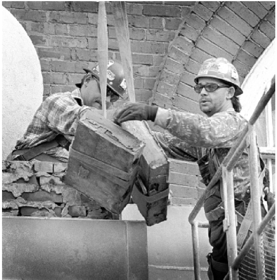
Brian Norton (l) and Richard Hartwig of Tupelo-based Pryor and Frazier Construction Co. carefully remove a stone and brick facade on Lee Hall. Built in 1909, the five-story designated Mississippi Landmark is undergoing exterior renovations.
