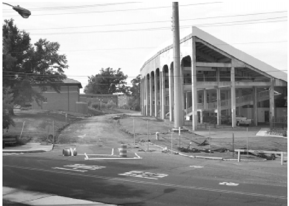
Construction crews recently removed pavement from Alumni Drive in preparation for the Davis Wade Stadium expansion of Scott Field. When completed during the 2001 football season, the $21 million expansion will add 50 skyboxes and 2,000 club-level seats to the east side of the field.
