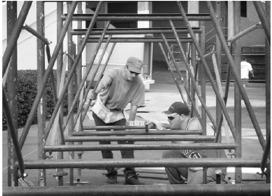
Preparing for the Bulldogs' first home football game on Sept. 30 against the University of Florida, a Birmingham contractor works on adding 22 rows of temporary seating to the end zone of Scott Field. The addition will accommodate 1,500 students during a sell-out season.
