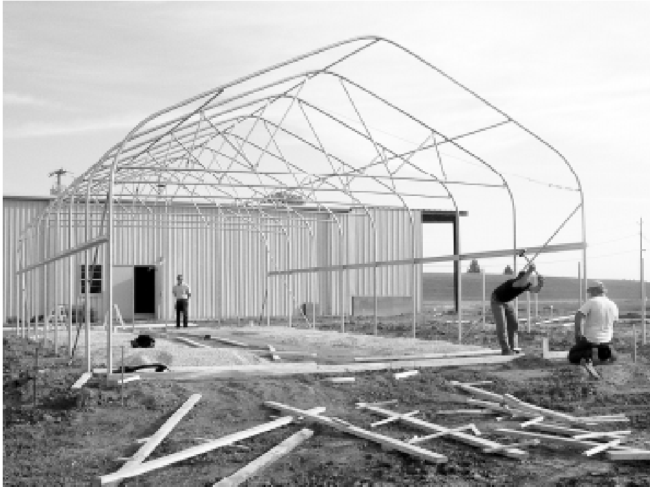
MSU research assistant Jacobo Caceres (l) works with Chalmer Wood and Dewayne Trahan, both of Louisiana-based Greenhouse Construction, to install a new greenhouse facility on the North Farm. The Entomology and Plant Pathology Department will use the structure for cotton, soybean, wheat, and turfgrass research.
