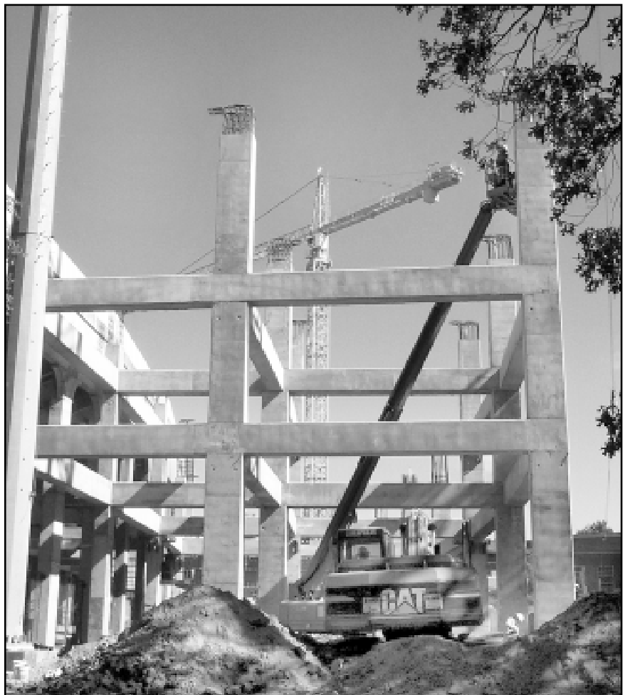
Work continues on the largest football stadium expansion project in MSU history as the east side of Scott Field begins to take shape. The $21 million renovation eventually will add 50 luxury skyboxes and 2,000 club-level seats to the facility.
