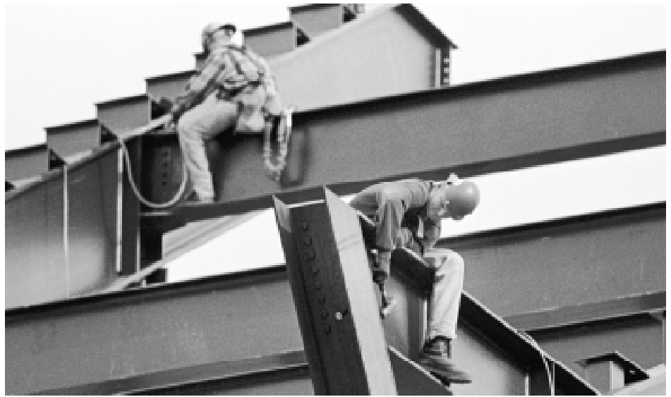
Workers pound in bolts as construction proceeds on the east-side grandstand addition at Scott Field. Approximately 35 percent complete, the renamed Davis Wade Stadium at Scott Field will have a capacity of some 52,000 football fans when work ends in the fall.
