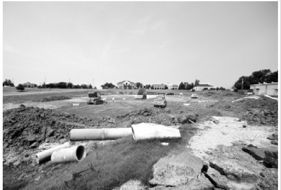
Site work is under way for a new landscape architecture building to be located north of Thompson Hall on Stone Boulevard. The 20,000-square-foot facility will take about a year to complete.
