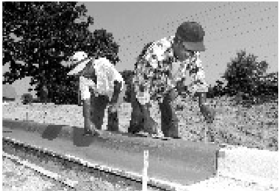
Moses Hall (l) and Willie Coleman, both employees with a local contractor, worked recently to shape curbing for improvements to Blackjack Road. The heavily traveled road is being expanded to three lanes from Locksley Way to Hardy Street.
