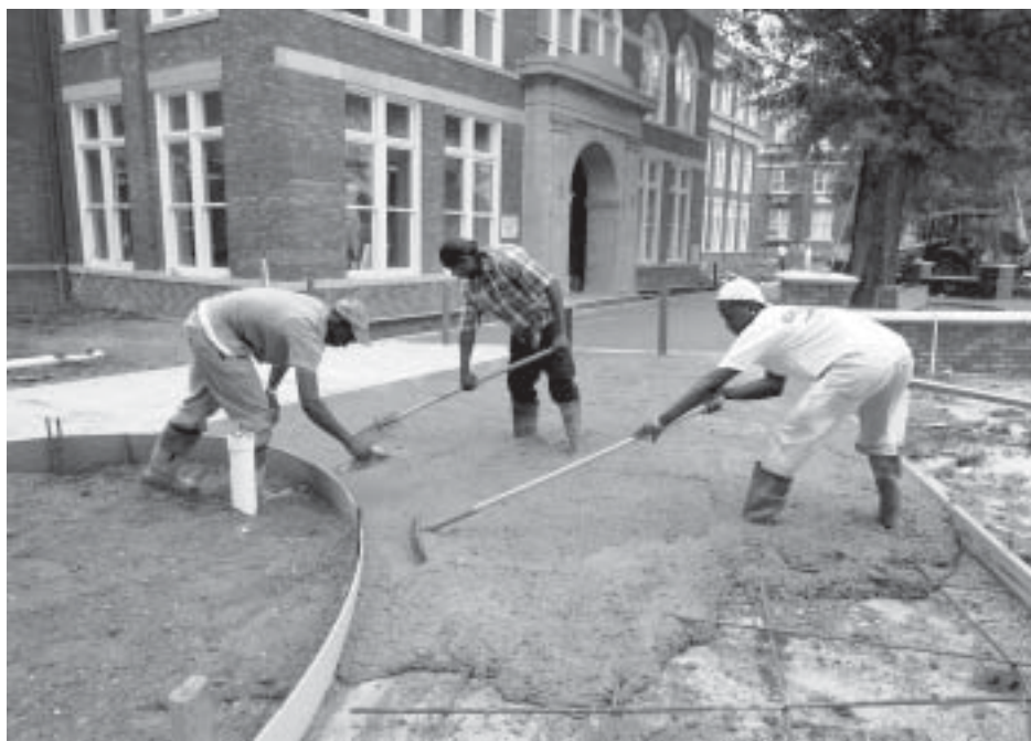
As restoration of historic McCain Hall continues, workers poured concrete recently for a new sidewalk. Concentrating on the task were (l-r) Charles Thompson Jr., Carlos Stepney and Demarkco Robertson, all of Columbia. A formal ribbon cutting for the refurbished engineering facility will be held Oct. 12.
