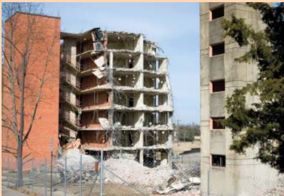
Demolition of Hamlin Hall is continuing into the new year as the seven-story residence hall becomes history. Only around half of the aging structure—built in 1966—remained standing as of Jan. 3.
