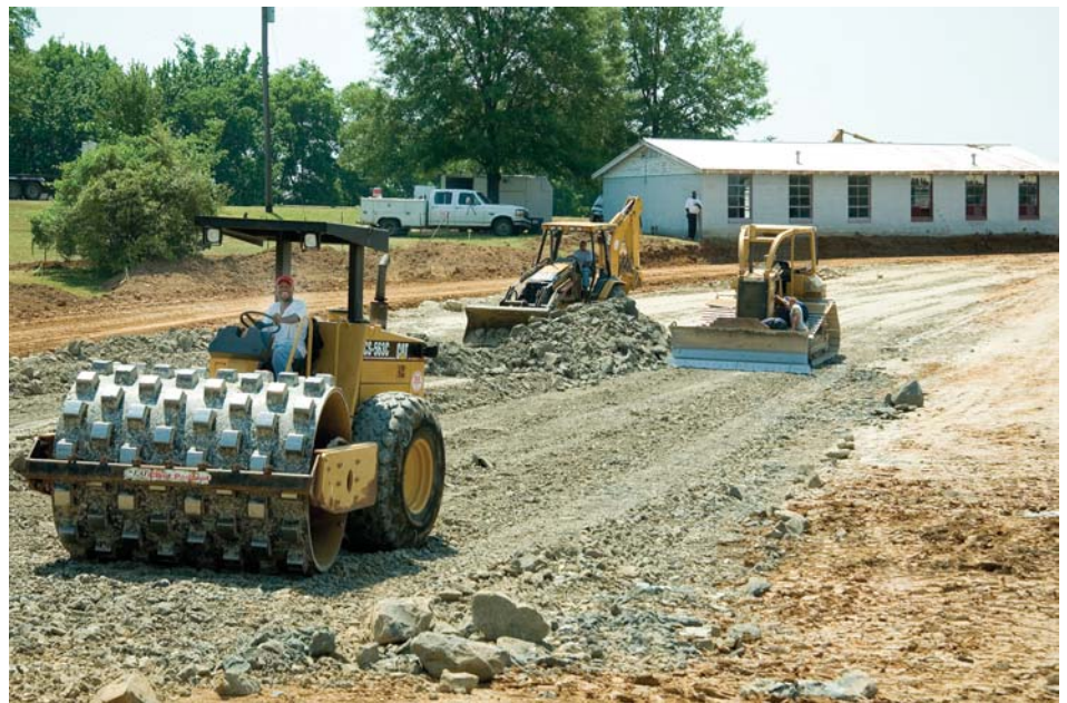
Heavy equipment crews worked recently on a new connector road that will link Bully and Stone boulevards.
