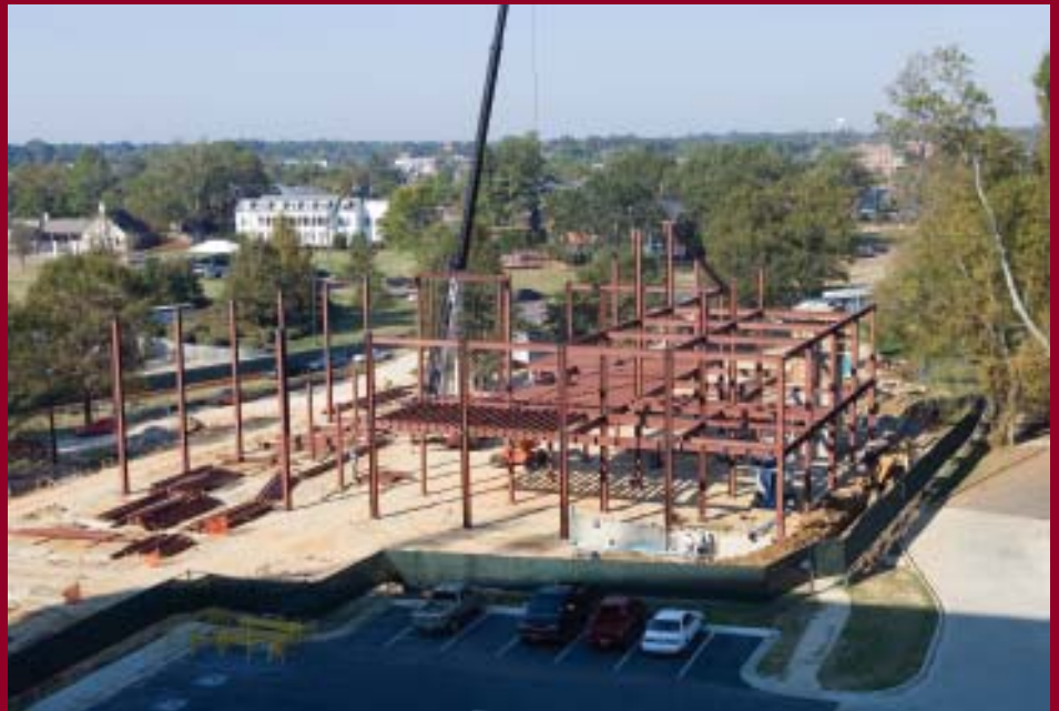
Generally dry fall weather has greatly aided construction of the Cullis Wade Depot on the west side of campus. Named in honor of its major benefactor, the nearly $9 million facility near the intersection of B.S. Hood and Creelman streets will house a clock museum, Barnes and Noble bookstore and other units.
