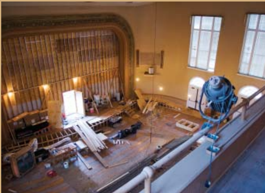
Renovation of the historic Lee Hall auditorium is under way as the spring semester begins. The 1,000-seat facility is being refurbished and enhanced, providing an improved performing arts venue for Mississippi State.
