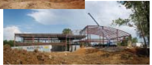
The $9 million facility housing automotive-related research is being built with state funds. Taking shape across the street, right, is the Powe Center for Innovative Technology, a small business incubator to be operated by Golden Triangle Enterprise Center and owned by the MSU Research and Technology Corp., which provided funding along with the Tennessee Valley Authority, the Economic Development Administration and the Appalachian Regional Commission.
